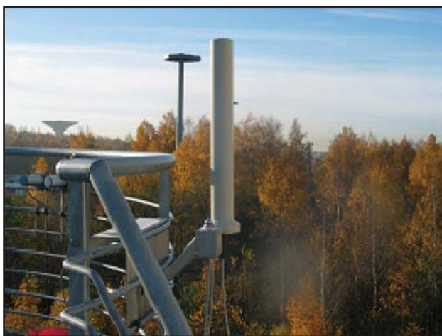
Fig. 9: Radiation dose rate monitoring station
